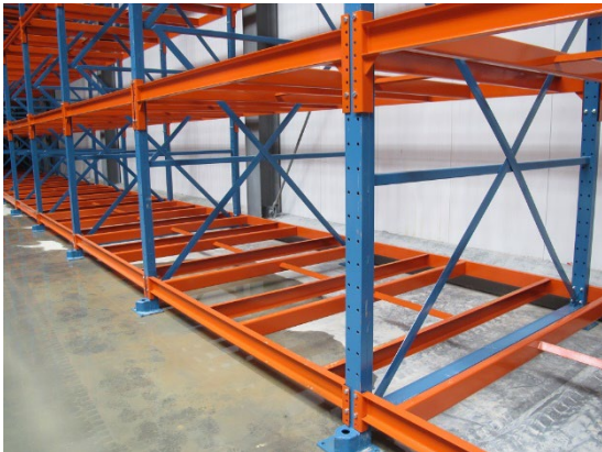
(I-2a) Pallet rack configuration
