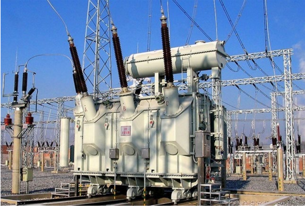
Figure I-2 LPTs: Installed large power transformer
