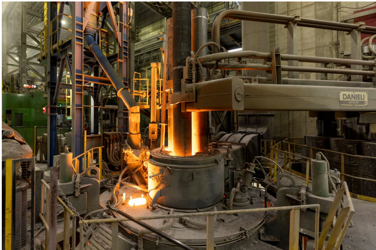
Figure 1.2 An electric arc furnace (three columns of LD graphite electrodes in the center)
